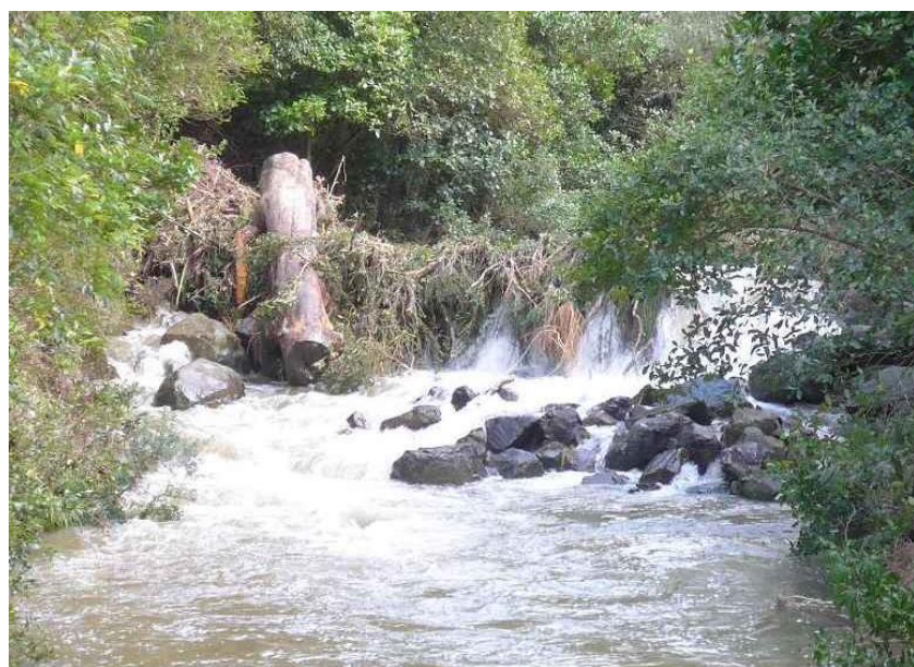
Debris trap after the 17 July flood, later cleared by Wellington Water Photo: Peter Reimann
